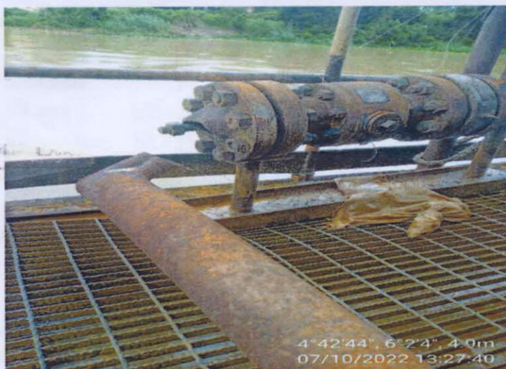
Fig 2. Affected Flowline Elbow
